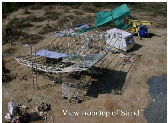
Stand and back crane aligned. Frame waiting for mirrors on the ground.
